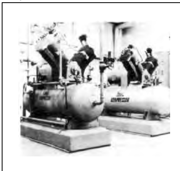
Fig. 10 Compressors "Red Cross", Bern
